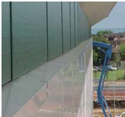
Misaligned cladding panels resulting from poorly installed secondary steelwork.
