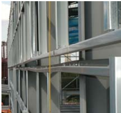
Poorly installed secondary steelwork.
