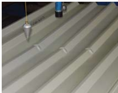
Figure 9. Failed pre-finished steel profiled sheet showing local buckling
