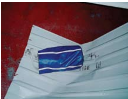
Figure 5. Failed non-fragility test where fasteners have torn through and the sheeting has failed
