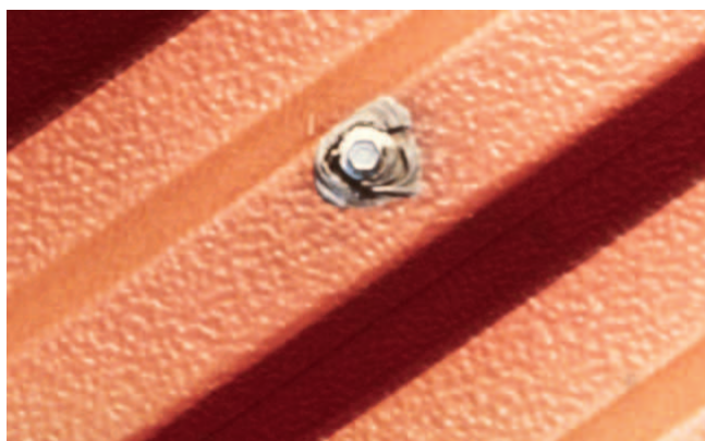
Damaged fastener on roof cladding
