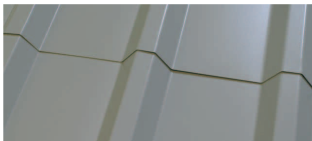
Cut edge on roof cladding
